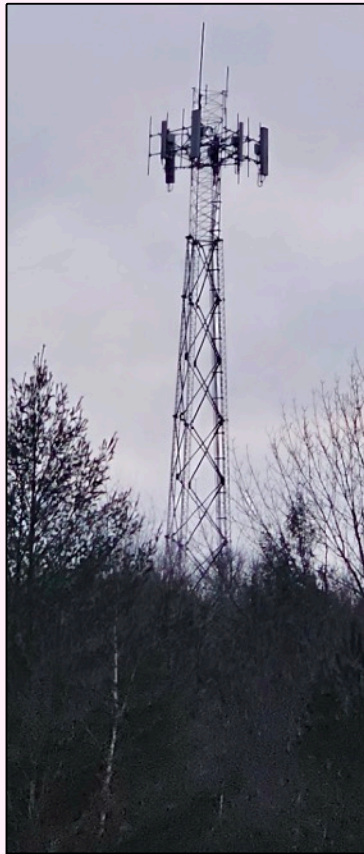
ITW's Fairfax Tower with T-Mobile Antennas
